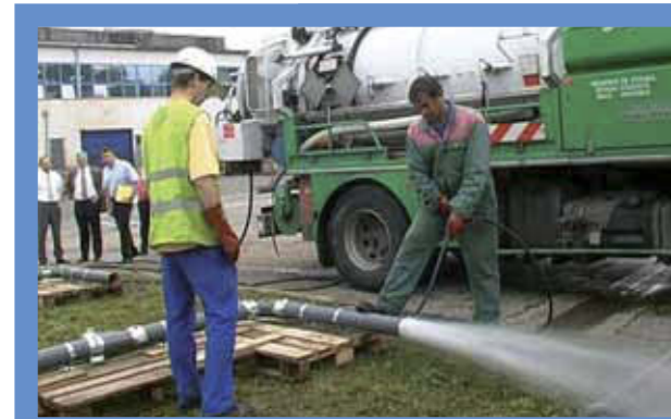
The S and Plus ranges, being assembled and anchored, have successfully passed a high-pressure jetting test: cleaning pressure of 120 bar from the pump, which means 100 bar at the nozzle outlet, without leakage or misalignment.
